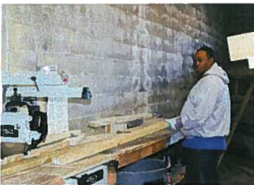
Jamaal Davis cutting materials for ramps during Martin Luther King day service project
