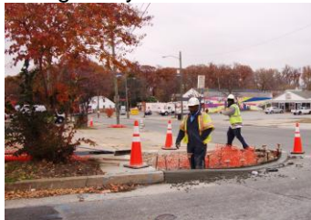
Workers put in first curb cuts in Nov. Photo Credit/ Frances Stanley
